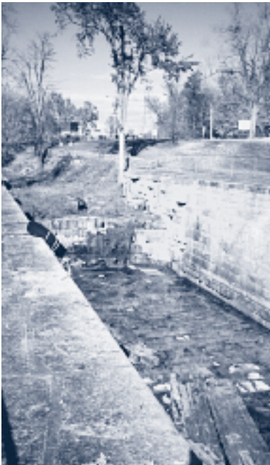
Important conservation work is required to protect the historic character of the Carillon Canal.
